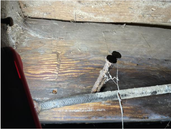
Ground-floor joist containing hewing marks. These timbers are in excellent condition, however immediate intervention is required (see next image).
